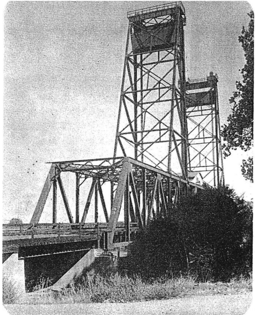
THE MOSSDALE BRIDGE that originally carried Central Pacific trains over the San Joaquin River east of Tracy in 1869 still stands today. The bridge has been strengthened and beams welded solid, but its basic structure remains the same.
